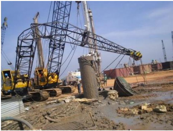
Gambar 55. Jib Crawler crane Patah
